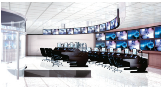
Monitor room in new building (23 Lac Trung Street, Hanoi)
