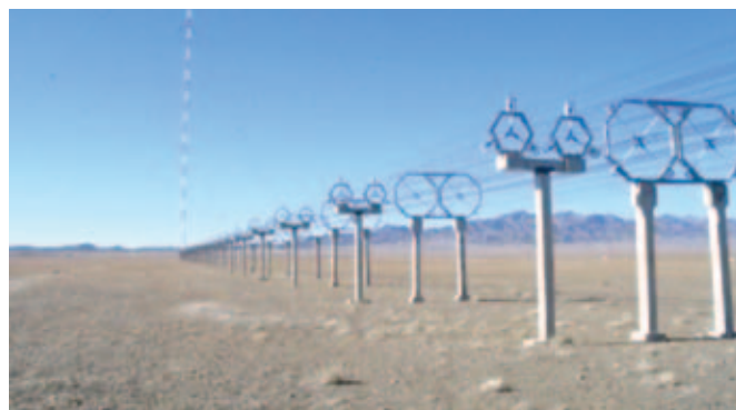
Feeder for LF antenna
