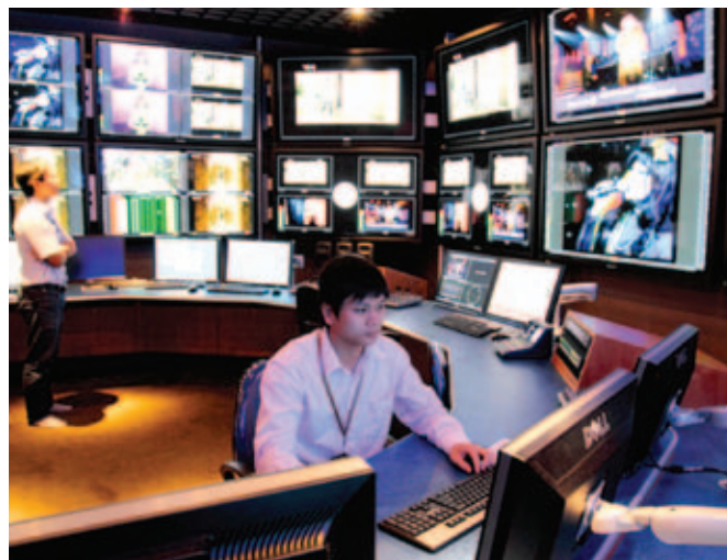
Figure 4: Network Operation Center (NOC)
