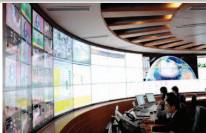
Figure 3: Network Control Center (NCC)
